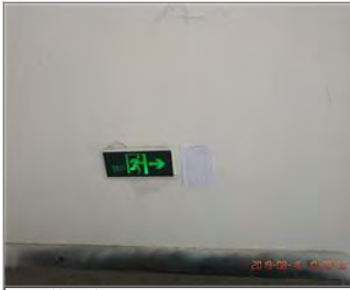
Photo of fire safety equipment evacuation sign.jpg
