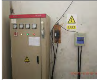
Photo of non-conformity NC No safety cover for parts of electric boxes.jpg
